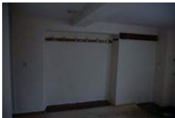
Fig.49 Blocked opening G5
