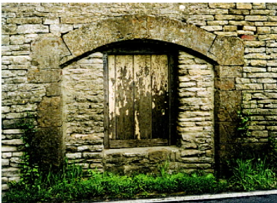
A fifteenth-century opening on the south elevation of Clifton Mill on the roadway—formerly the Burford to Buckingham Turnpike
